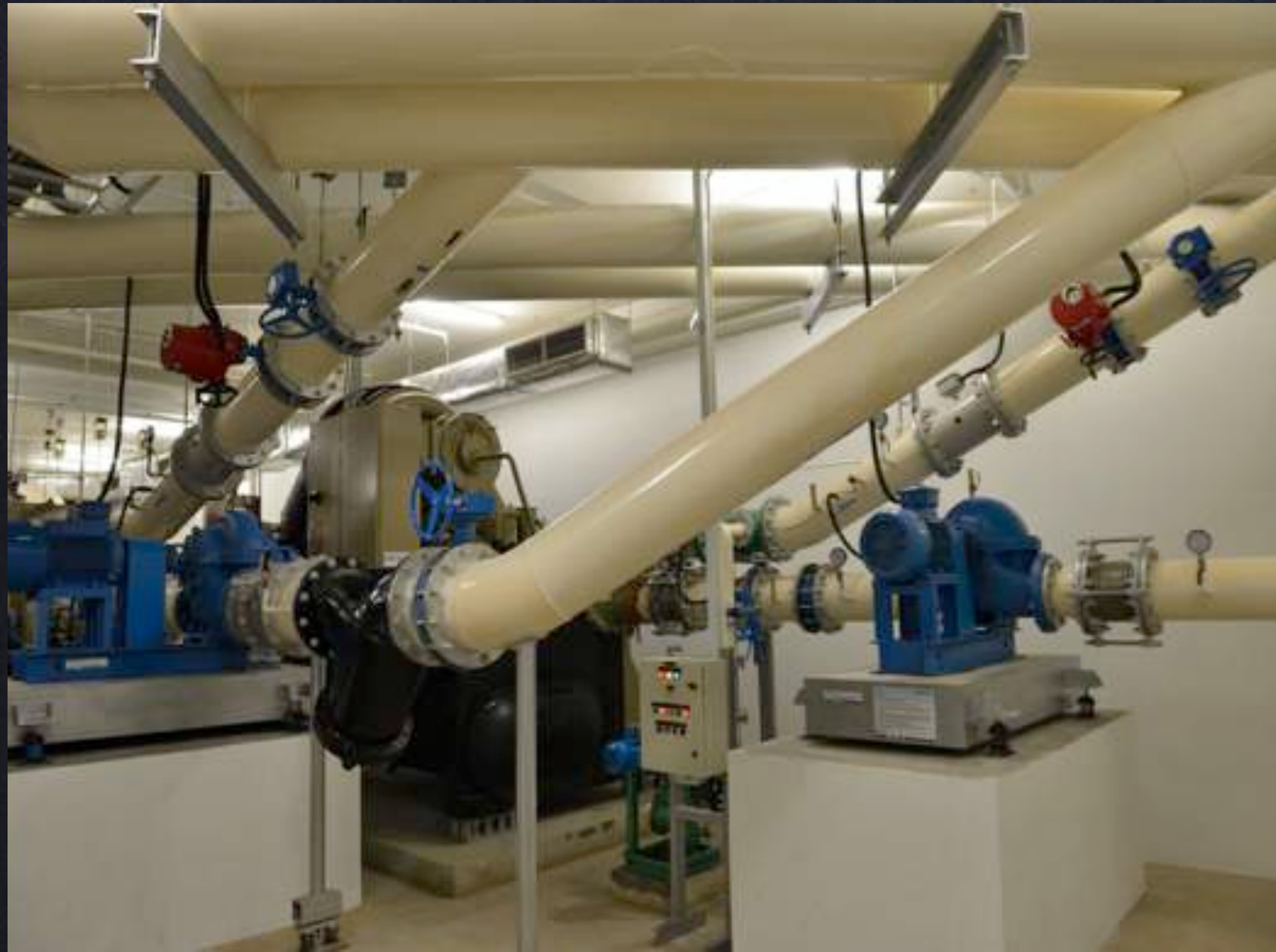
Big pipes, small pumps
